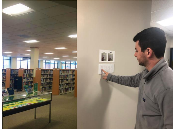
Interior LED Lighting Upgrade Project Advanced Plug Load Control Project
