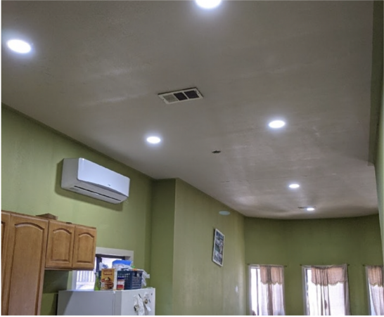
Above: Building Electrification in West Oakland
